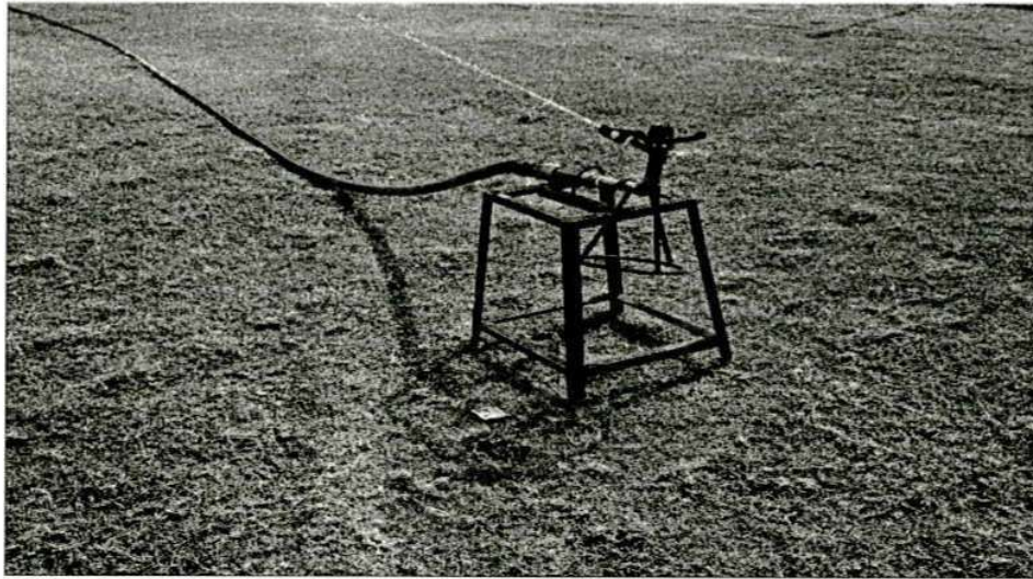
Figure 2.3:-Water Sprinkler system in university lawn
